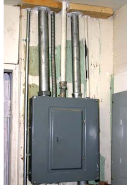
No more exposed wires!
