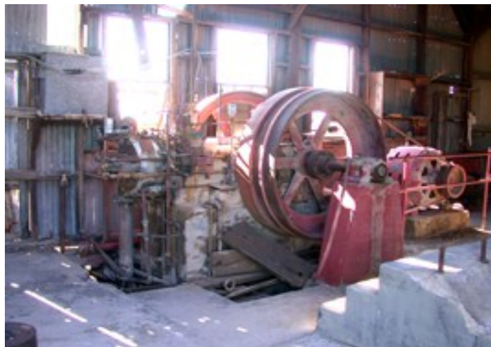
Inside the power plant, which also served as a machine shop. All tools and machinery still in place.
